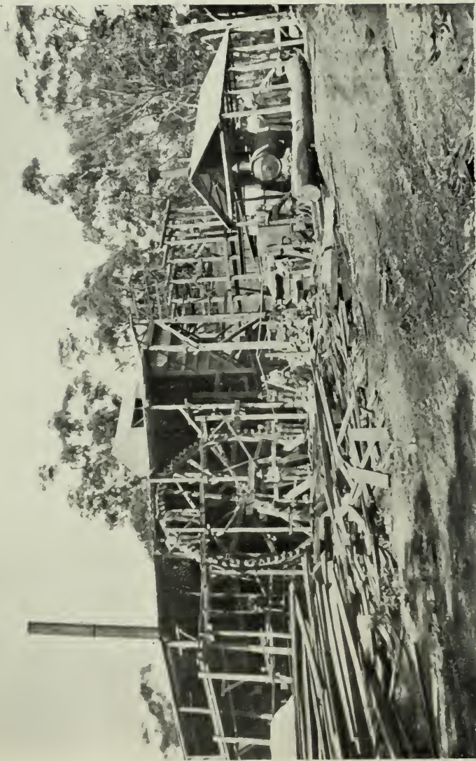
Mrs. J. Shannessy, Rockvale Wolfram Company's Battery and Concentration Plant (under construction). Tungsten near Torrington.
